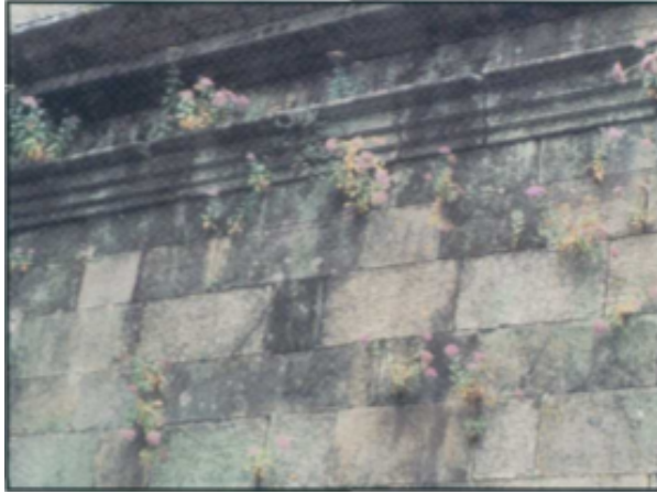
Figure 5. Formation of gypsum crystal structures in marble under shelter. Pollutants captured in the crystals create a blackish colouration, and cracking allows for plant life to grow through structures (McGee, 1995).
